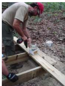
Ranger Ken works hard on building a new bridge that will go along with a new area of the PMT.
